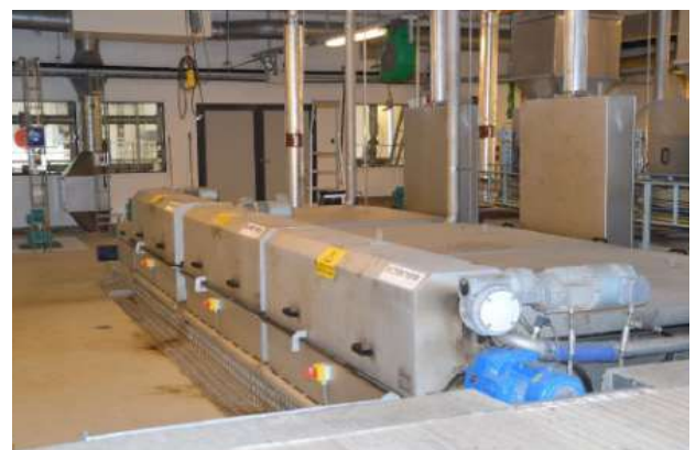
Three of the six SFK600 Salsnes Filters installed at the Plant
