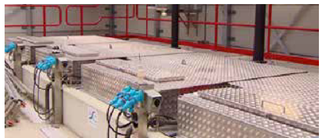
Four of the eight SFK600 Salsnes Filters installed at the plant
